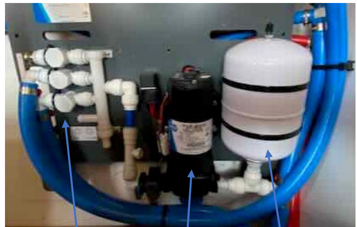
Tank Selection Valves"
