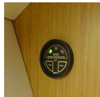
LPG leak detector
