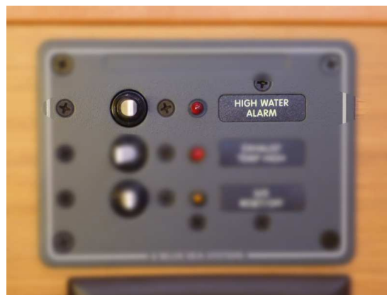
Bilge high water alarm
