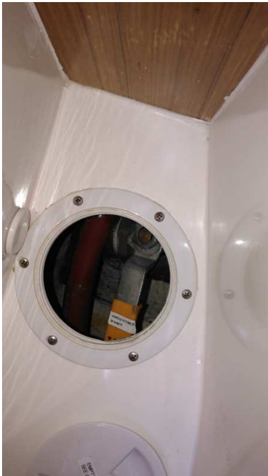
The valve handle is visible below the cover
