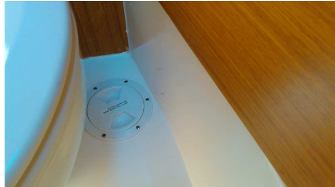
The ball valve is located under an inspection cover outboard of the aft toilet
