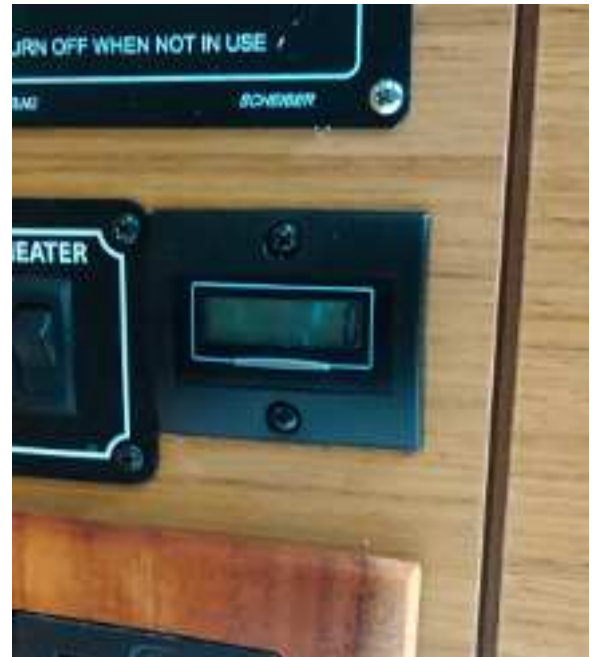
By-the-gallon water meter
