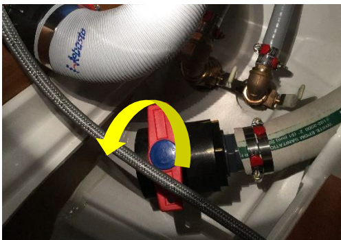
Forward Head Gravity Valve Under the sink.
