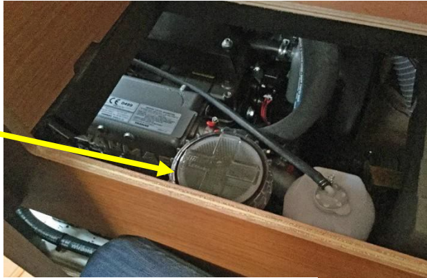
Raw Water Strainer- View from Port Aft Cabin Hatch
